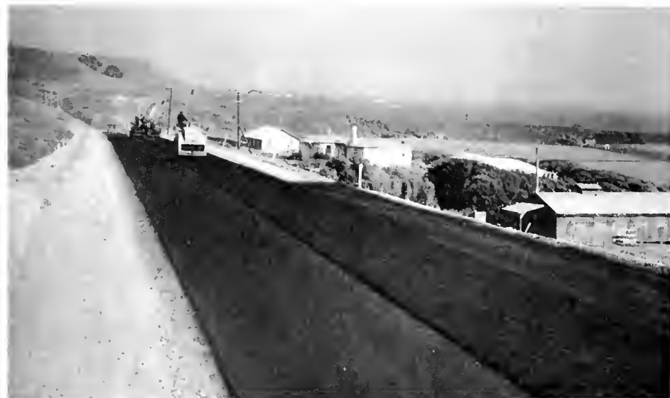
Looking south from north end of job, showing new shoulder, first course of plant-mix surfacing, and second course being placed and rolled
